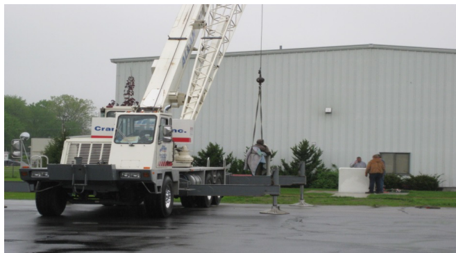
Installation of WWII Pilot Statue and large hangar that borders Aviation Heritage Park
