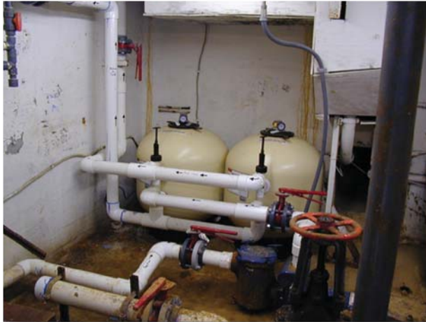
Chlorine storage and feed area
