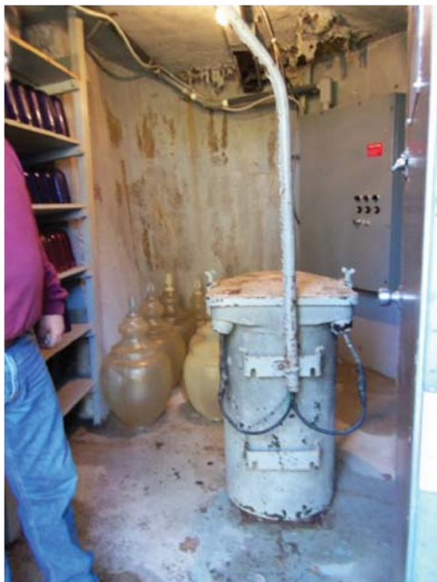
Step Down Transformer in wet vault under Cascades
