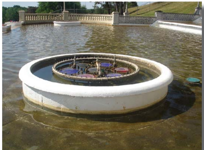
Existing spray fountain (1 of 6)
