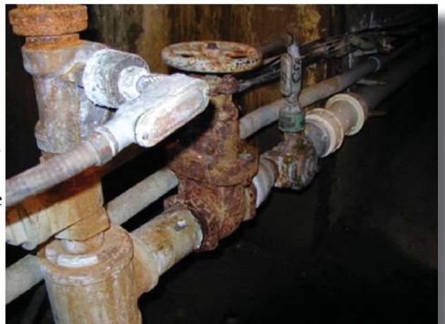
Severely corroded tunnel piping and valves
