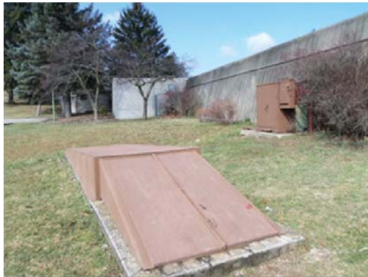
Entry Point to Underground Mechanical Room
