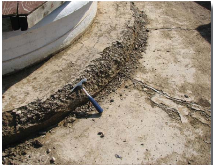
Concrete Deterioration at Upper Pool
