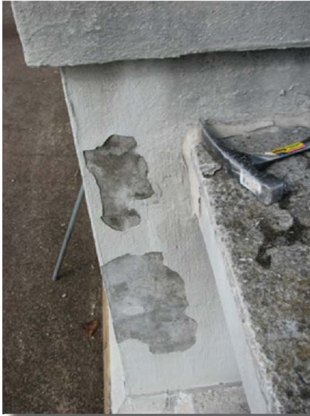
Existing Concrete Coating, Failing in Numerous Locations
