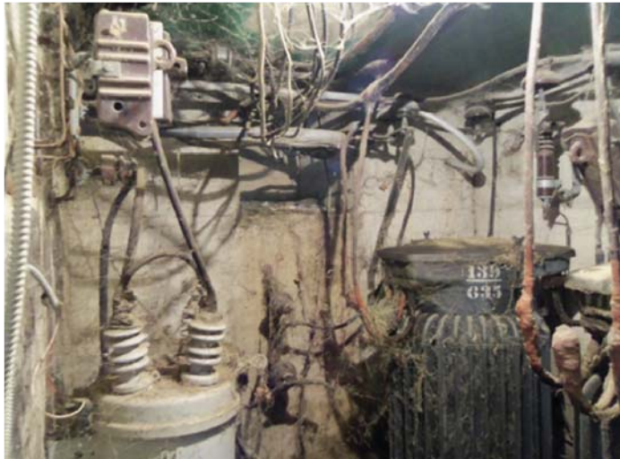
5,000 Volt gear in Vault
