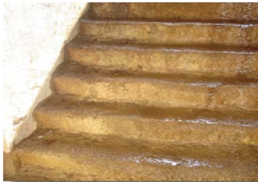
Wet, uneven, failing existing stairs
