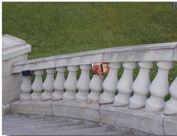
Corroded Stair Lighting
