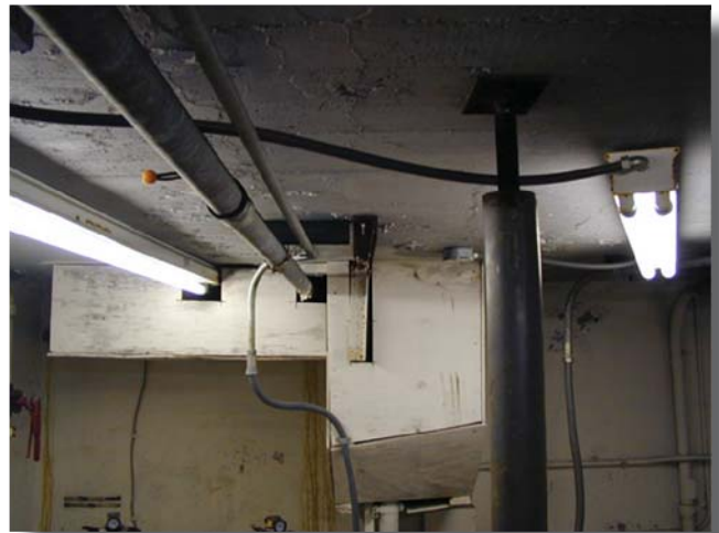
5,000 Volt connections covered by plywood
