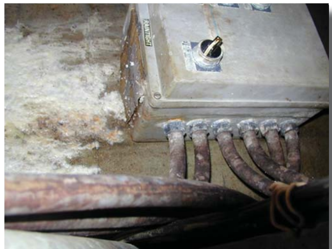
Corroded Electrical Equipment in Tunnel (Wet Environment Typical)
