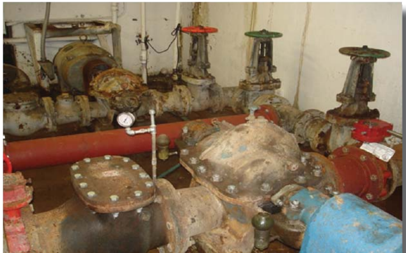
Aged mechanical equipment in underground vault
