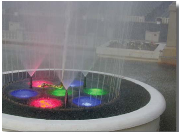
Fountain with clogged nozzles in left foreground
